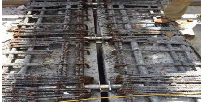
Installation of the DSD and local reinforcement for high shear load transfer
